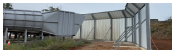
At NPM, a range of noise reduction strategies were used, including the installation of an acoustic wall.
